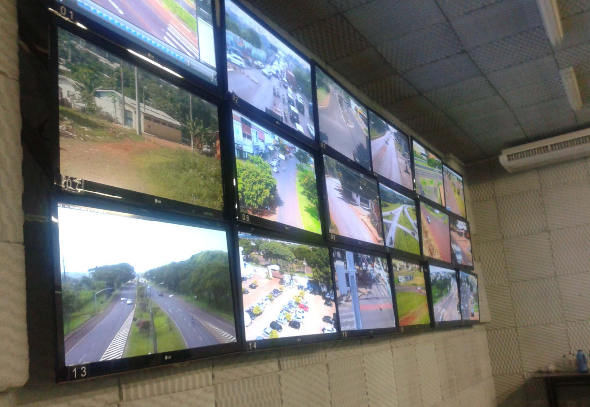
Central Monitoring Station
